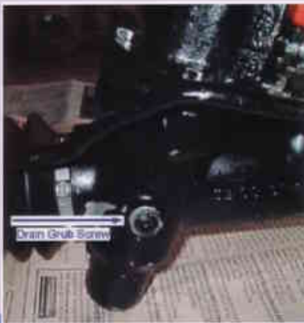
Above: The leaked fluid drain grub screws.
