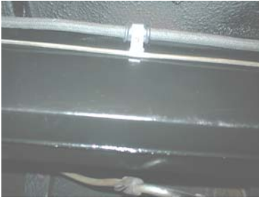
Detail of the chassis mounting of the mail battery cable and brake pipe in the Silver Cloud
