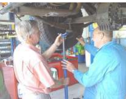
Don Positions The Jack Stand To Support The Base Of The Spring
